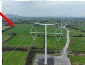
National Grid substation and HPC connection pylons
