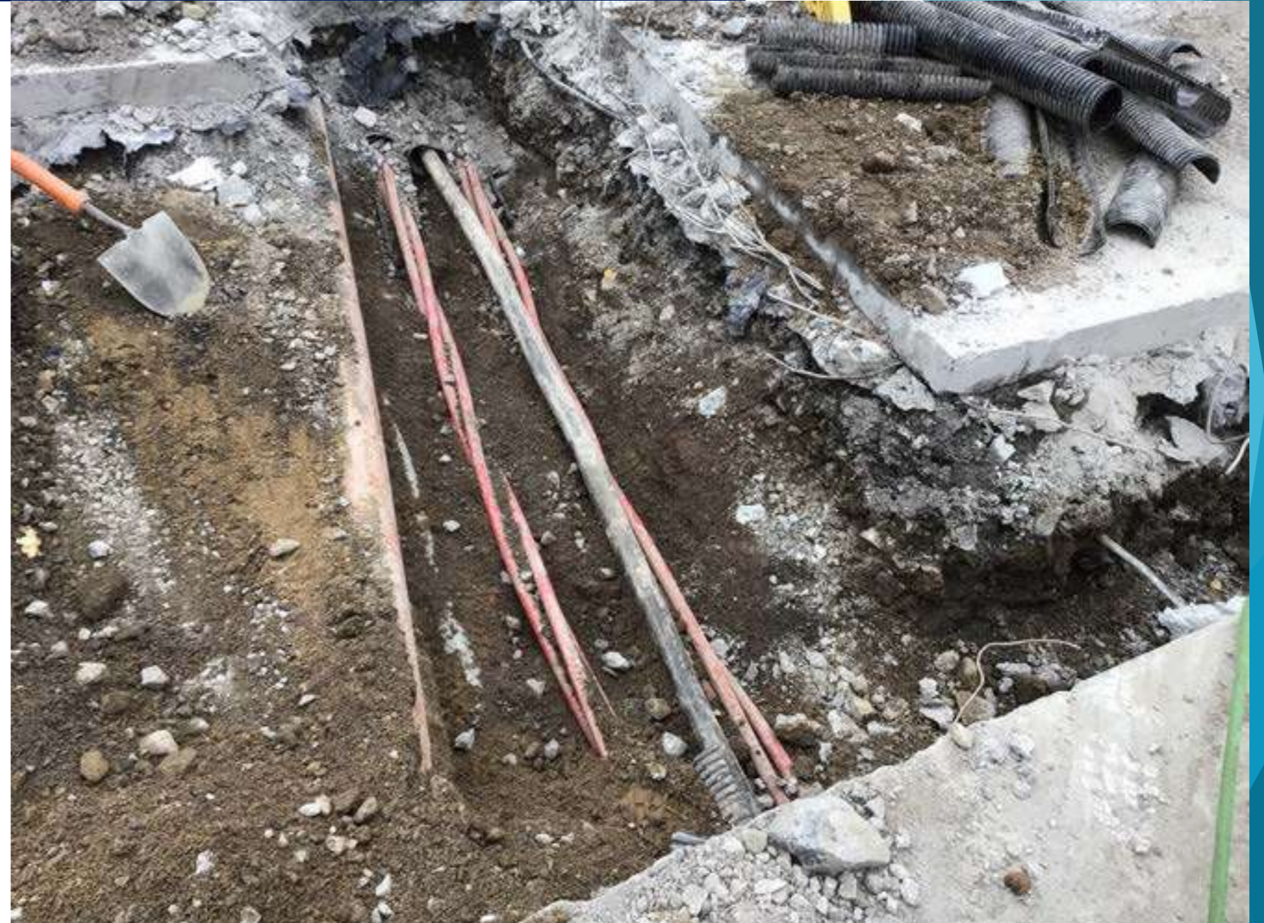
2 HV Cables, 1 LV Cable, Street light Cable, BT duct and drain pipe under reinforced concrete
