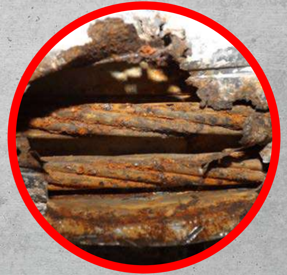
Grouting Defect Heavy Corrosion
