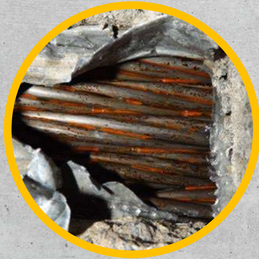
Grouting Defect Light Corrosion
